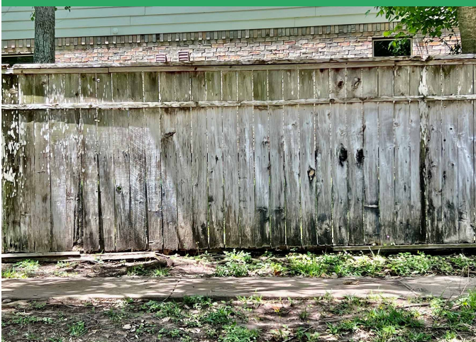
SIDE FENCE IN NEED OF REPAIR
